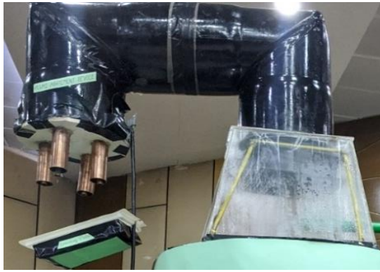
Figure 5: Photograph of water collection system.
